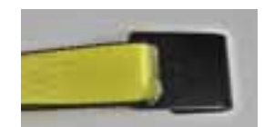
End hardware damage
