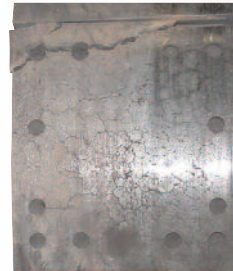
Cracked competitor's lining
