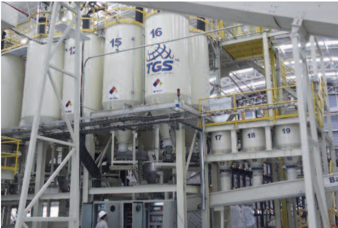
Automated weighing system ensures batch-to-batch consistency
